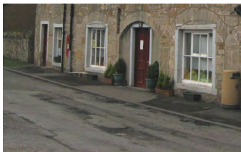
Damaged road surface in front of the Sutlery
