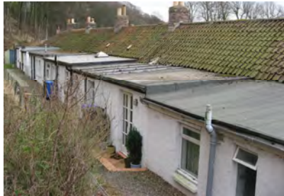
The flat-roof extensions at the back of North Row, seen from the elevated garden plots.
