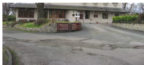
Patched road surface in front of the Elgin Hotel
