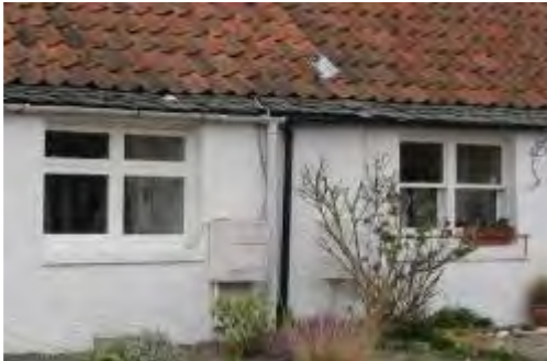
Compare the original style windows on the right with replacements on the left. Note also the two prominent meter boxes.
