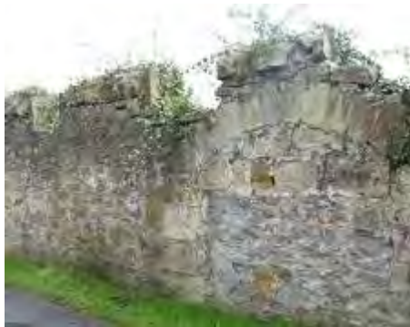
Crenellation to top of rubble wall opposite Limebank, overlooking the site of the former limeworks.
